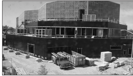
A building committee helped oversee a new facility for Fountaindale Public Library, now under construction and set to open February 2011.
