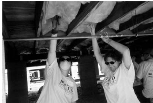
She also worked with a team to install insulation under the home, which is elevated.
